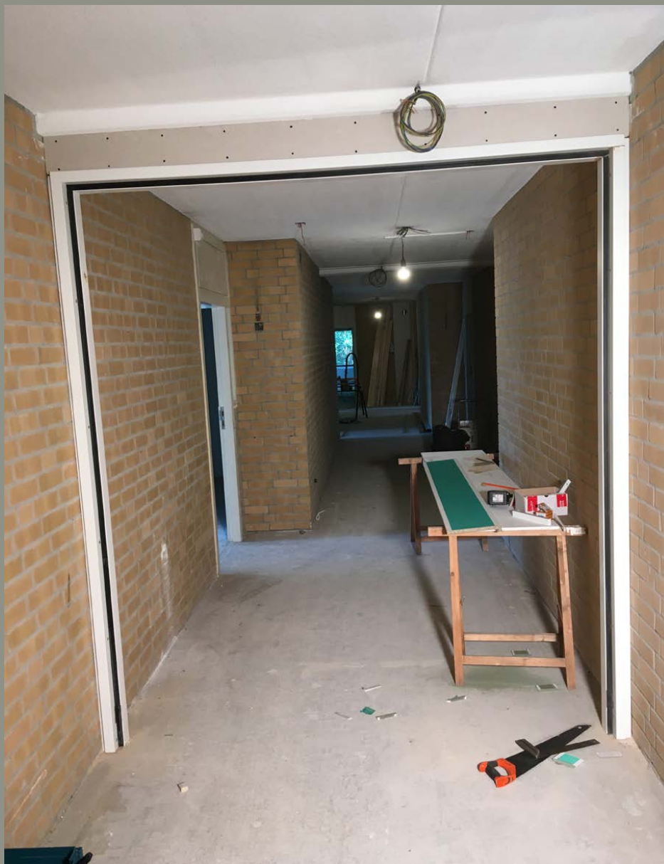
Extra brandcompartimentering in de corridor.
